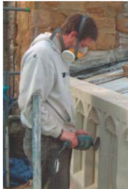
Above: Final finishing and adjustments were made to the newly placed stone work.
